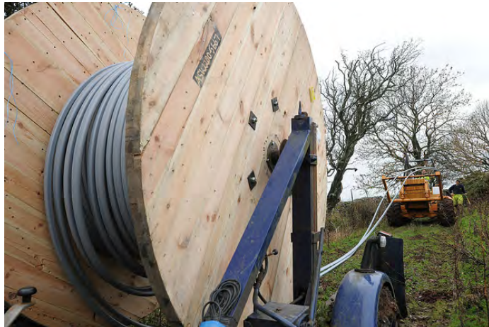
Fiber optic cables being installed. (PHOTO: Johnnie Pakington for BT, Flickr CC )
