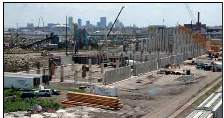
A view of the facility by Marcus Construction (Photo from the West Central Tribune)
